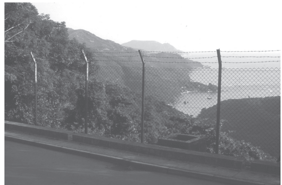
Figure 13. Chain link fence at the crest of a roadside fill slope in a scenic area
