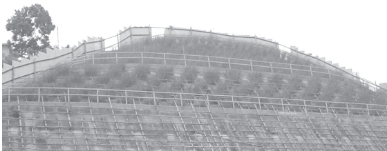
Figure 11. Vetiver grass cuttings in pockets and strips on the upper two batters of a 40° – 45° soil cut slope
