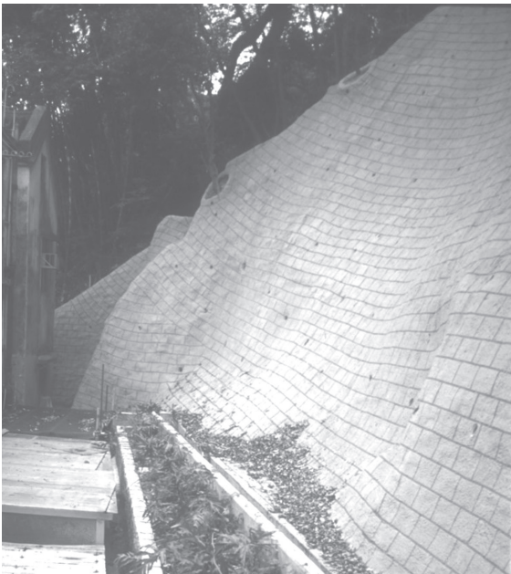
Figure 9. Granolithic spray coating used to create a stone-block effect on a shotcreted soil cut slope
